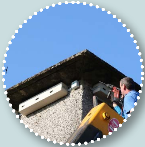
Genesis Swift Boxes installed with caller system at Trim Town Hall
