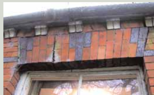
The lintel in this late nineteenth-century building needs urgent attention. The cracked brickwork and depressed head of the window indicate that it has failed. The brickwork appears to be saturated, which will worsen the structural problem
