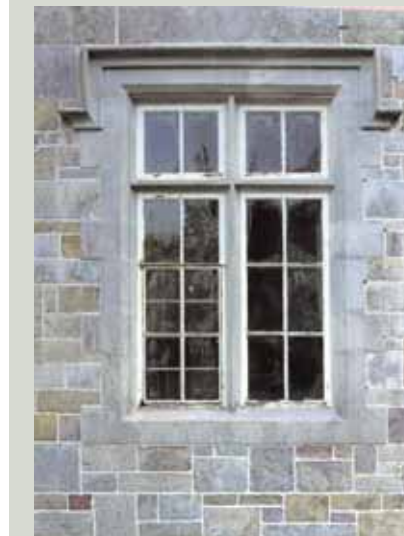
A number of signs of corrosion are visible on this window, especially on the casement (lower left of the window). This may require specialist repair. Elsewhere paint is failing, but the metal does not seem to be badly affected yet
