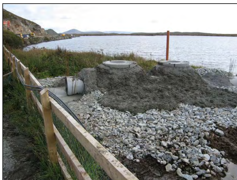
Plate 1.9 – Pollution Bypass Separator (Example at N59 in Connemara adjacent to Derrylea Lake SAC)
