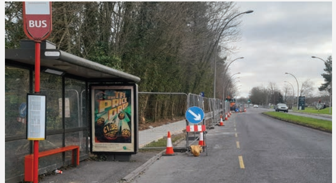
New bus shelter and associated works opposite the Skycourt Centre Shannon. New bus shelter and associated works opposite the Spring Hotel In Ballycasey Shannon.
