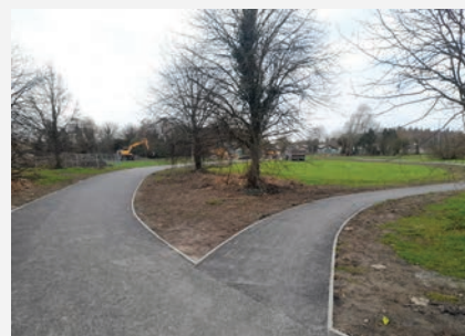
Works are progressing well on the Active Travel project in the Ballycasey Park Shannon. The works include new footpaths, paved areas, new public lights, and new street furniture.
