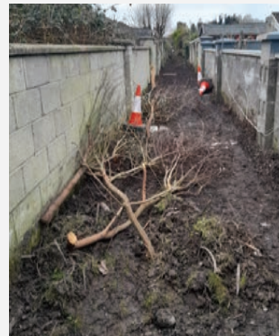
General maintenance, removal of overgrown brush, removal of waste material, and repairs to stormwater manholes at Tullyvarraga Shannon.
