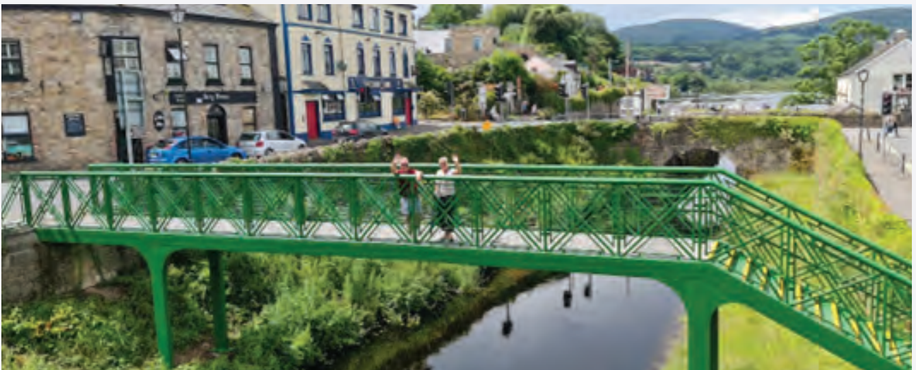
Photo of completed repairs, refurbishment and painting of 'The Green Bridge', Killaloe.
