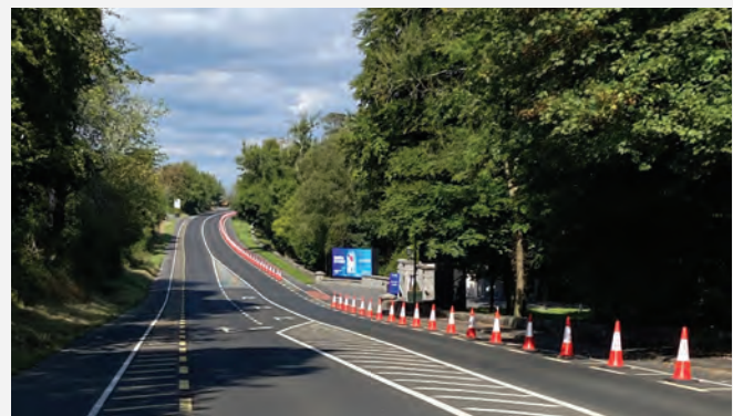
Work undertaken by Shannon Municipal District in preparation for the KPMG Women's Irish Open included coning of the R458 cycleway, north direction.
