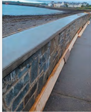
Wall capping to a section of sea wall at Cappa. A section of the stone façade of the wall had previously come away from the RC supporting wall. These works are funded by the Climate Change Adaptation and Resilience Works scheme.
