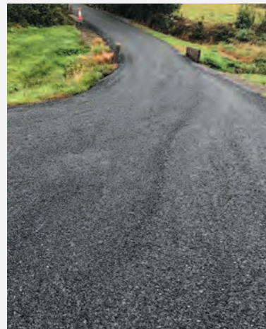
Preparatory works for road reconstruction and resurfacing at Kiltumper. These works are funded by Kiltumper Wind Farm.
