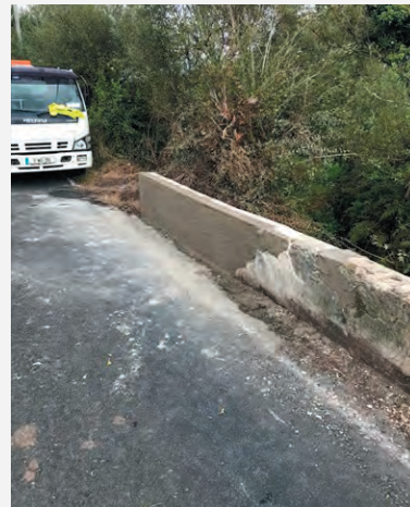
Repair of a bridge parapet near Cree. The parapet was struck by a car.
