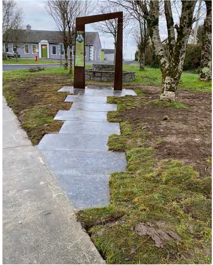
Further progress on the Fáilte Ireland Discovery Trail Project with the installation of the Doorway in Corofin.
