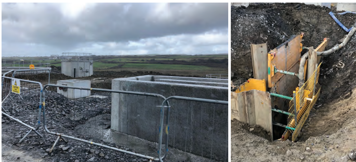
Above left: Tanks in place at the WWTP in Liscannor. Above right: Excavation for manhole at the pump station in Liscannor.
