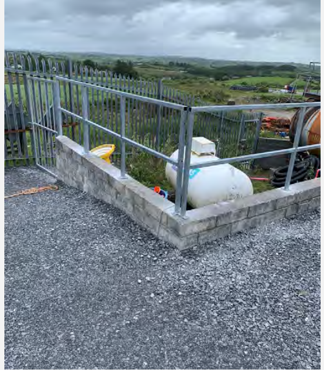
Safety railing around gas tank, Cliff Quarry depot
