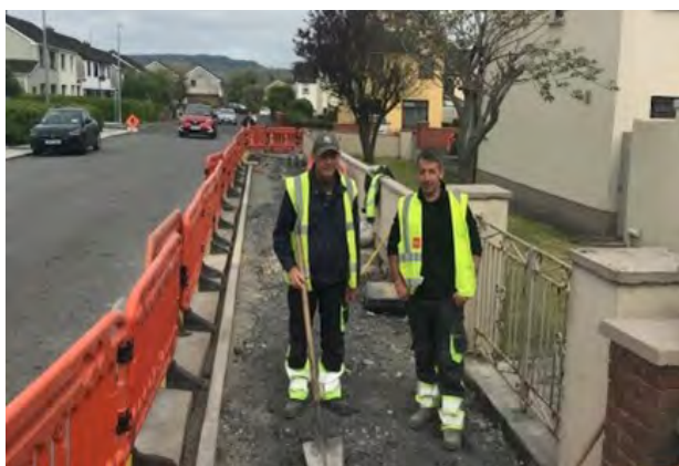
Pictured: Mike Meehan and Hugh Ward from the team in Shannon Municipal District delivering a new footpath in Shannon Banks during May and surface dressing in Meelick.
