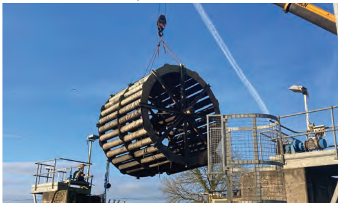
Stehlar Wheel at Tulla WwTP.
