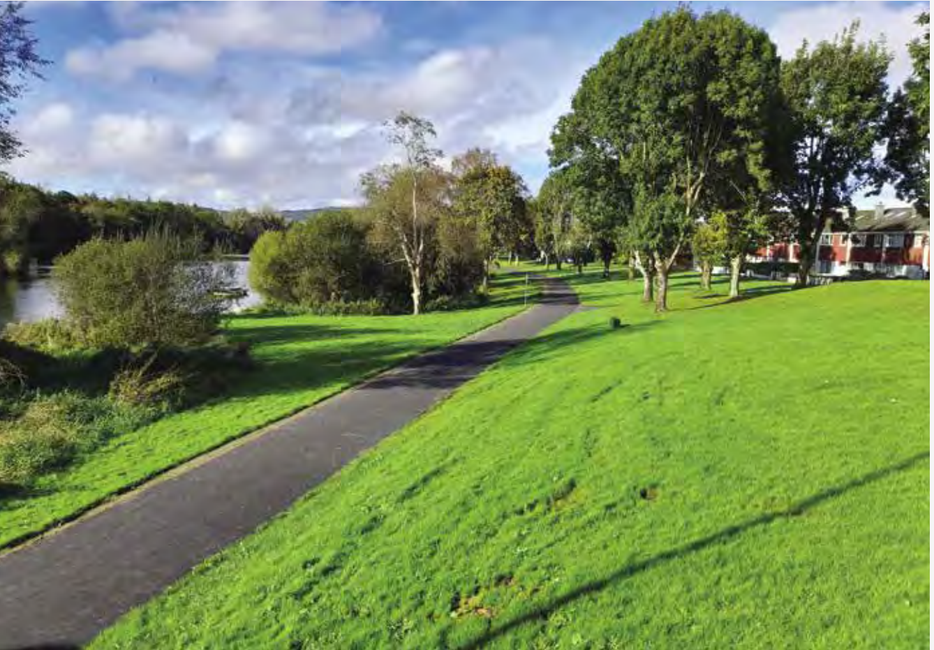
Pictured: Works carried out in Shannon Banks under the NTA Active Travel Fund.
