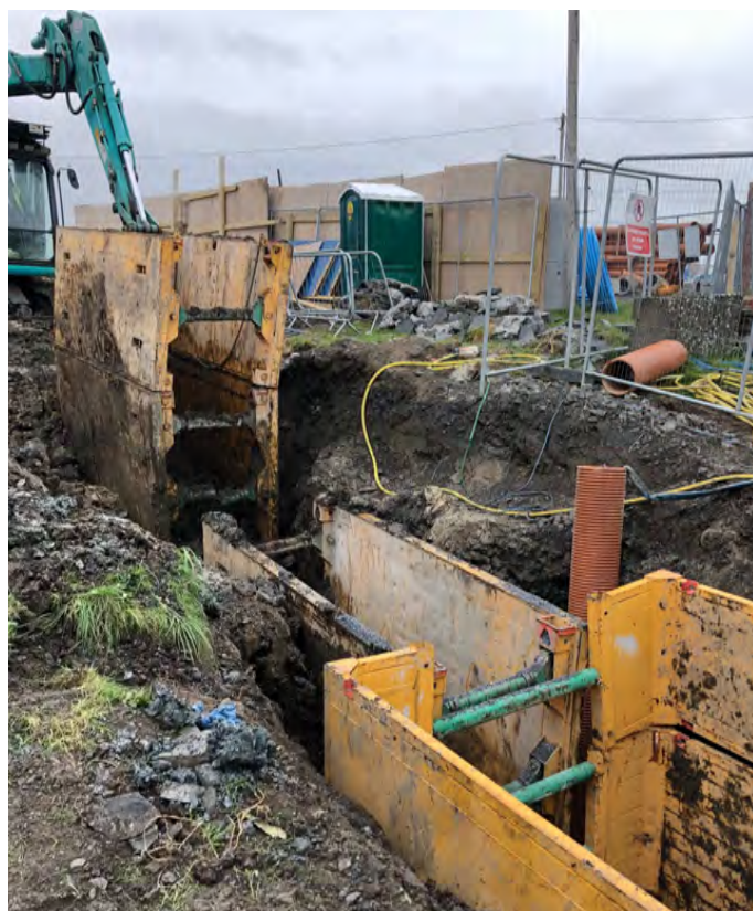
Liscannor Pump Station.
