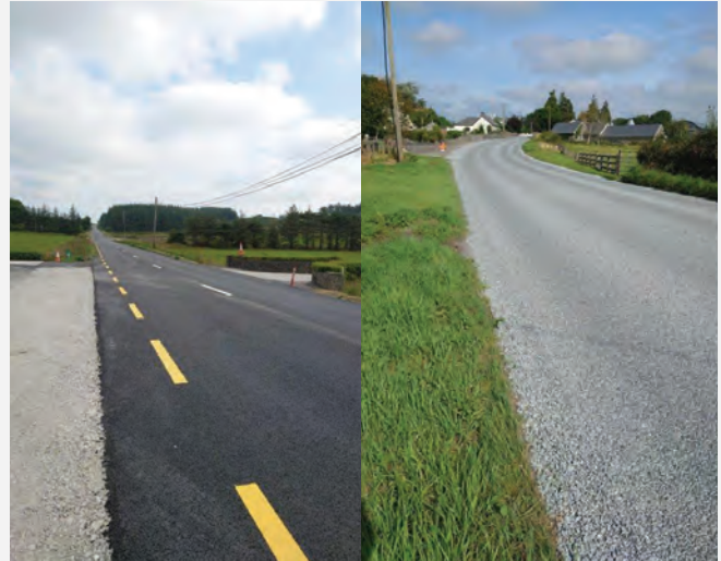
Above left: N68 Caherea to Lissycasey resurfacing currently underway. Above right: R472 Tiermaclane Surface Dressing.
