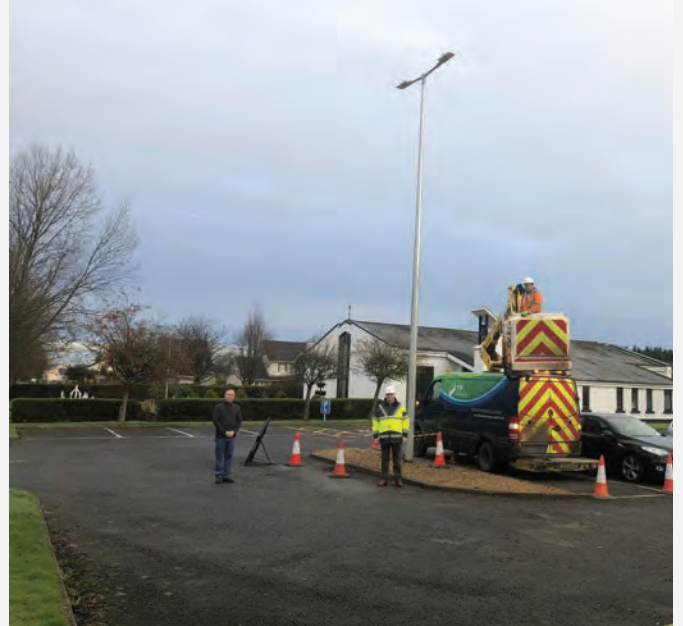
Lighting at Shannon Church.
