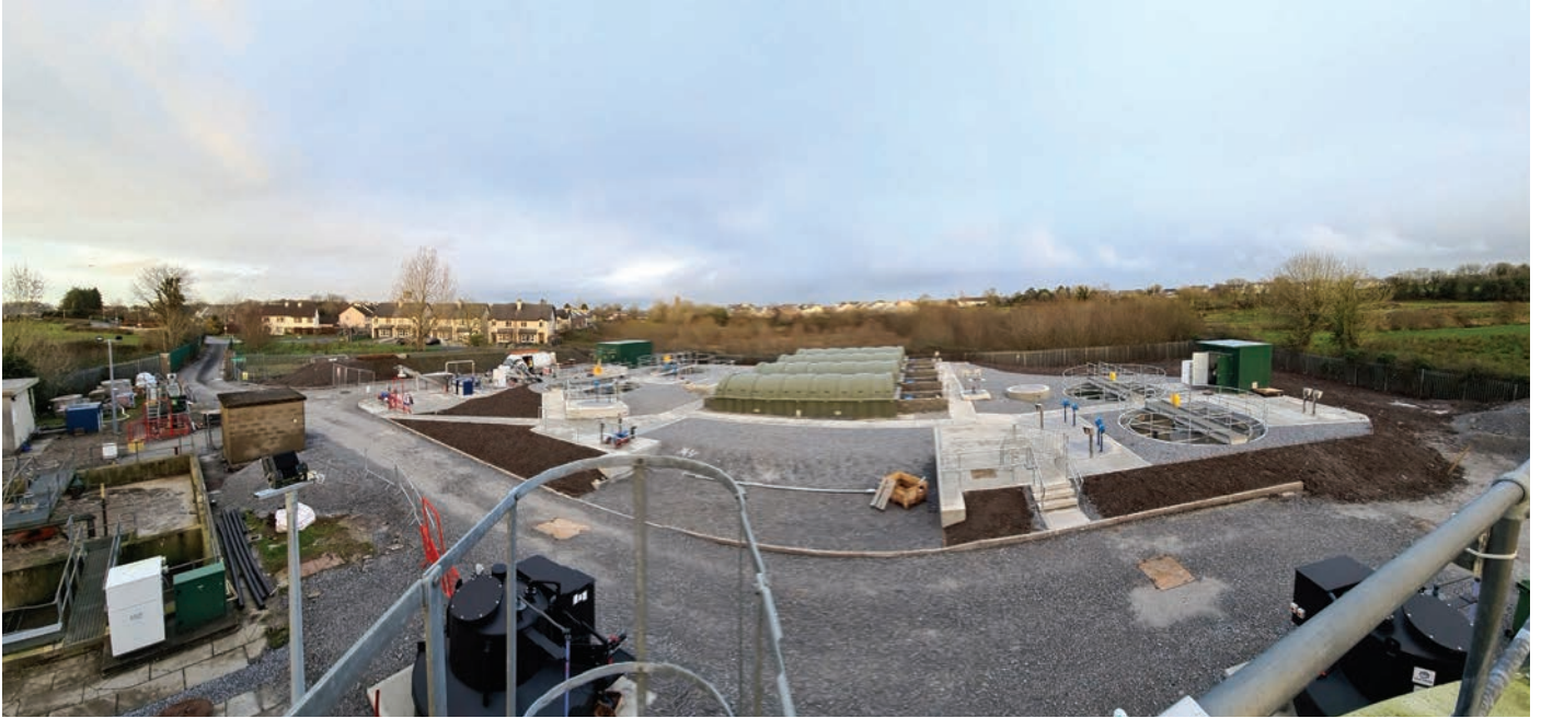
The new upgraded Quin Waste Water Treatment Plant which is nearing completion.
