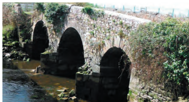
Latoon Bridge works - before repair.
