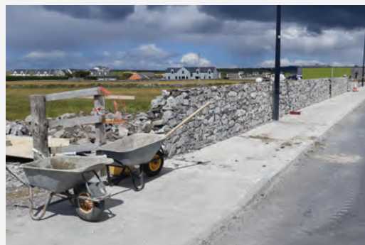
Works are due to be completed on the final phase of footpaths from Fitz Cross to Fisher Street, Doolin.
