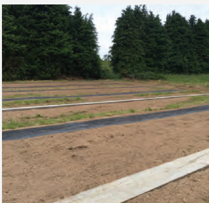
Plinth and path construction at Ballycannon have been completed by local contractor Syl O'Connor.
