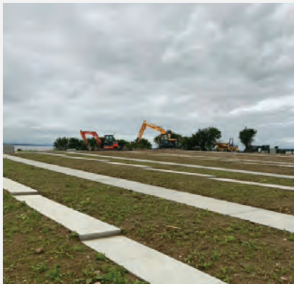
Work is progressing well on the major extension at Illaunmanagh BG in Shannon.
