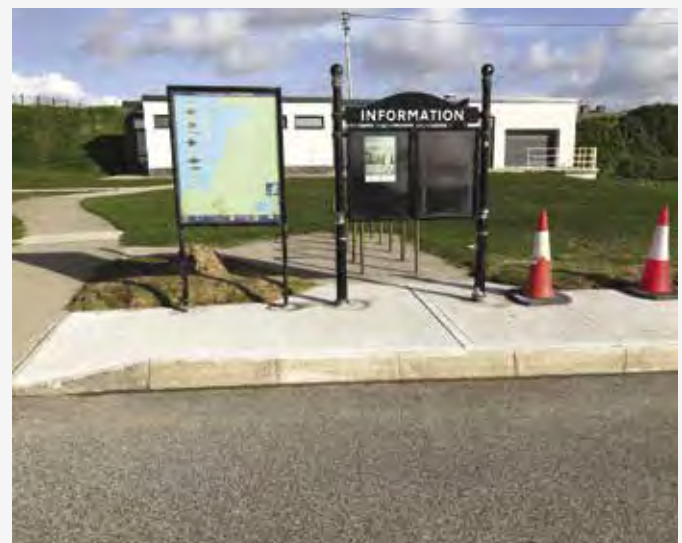
Works recently carried out by the WCMD in Spanish Point as part of the ongoing beach amenity improvement works.
