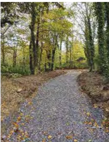
Off the N67: Entrance to Vandeleur Gardens, Kilrush. New section of path through existing forest.
