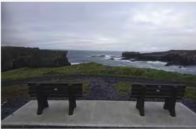
Works carried out at the Bridges of Ross by the West Clare Municipal District (WCMD) under the Department of Community and Rural Development's 2019 Outdoor Recreation and Infrastructure Scheme.
