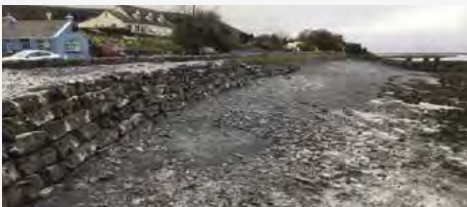
Rock Armour recently installed by the WCMD in Ballyvaughan Pier under the Department of Agriculture, Food and the Marine Fishery Harbour and Coastal Infrastructure Development Programme 2020.
